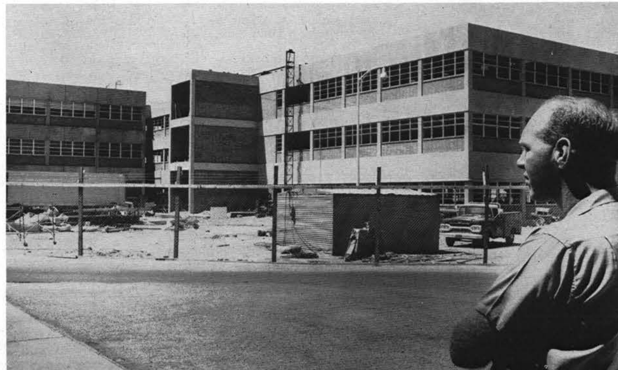
PROGRESS of construction of Bldg. 861, Phase II, is viewed by V. O. Kerr (4543-3), Plant Engineering project engineer. Completion date of the new building will be about Aug. 27. It will house laboratories and offices of the Research organization. Move-in of personnel should be complete by January 1962.
